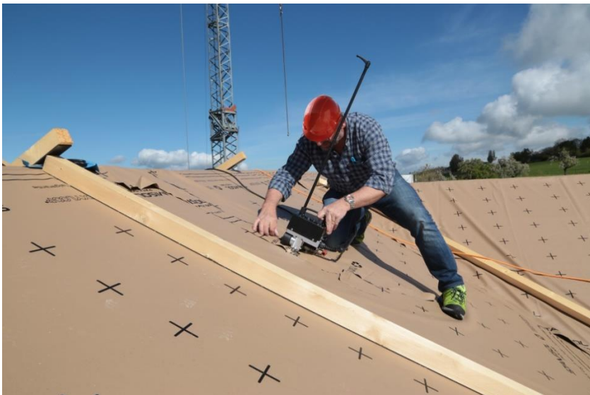
Outdoor welding of typical sub-roof membranes with close edge welding in Switzerland 2017.
